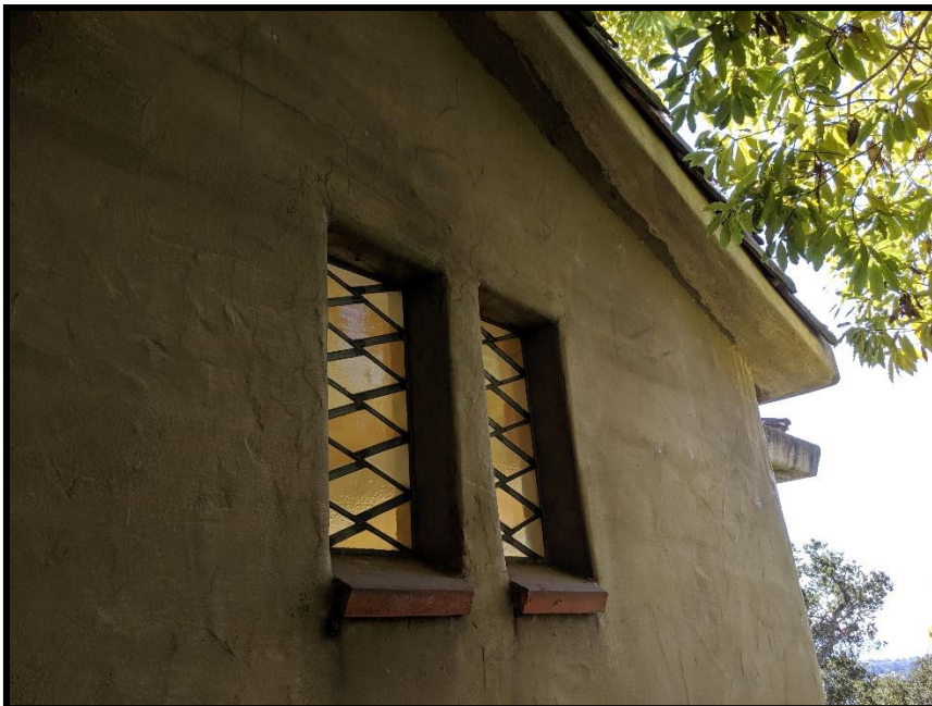
Figure 24: 4 Mosswood Lane - windows on north facade with leaded design in colored glass
